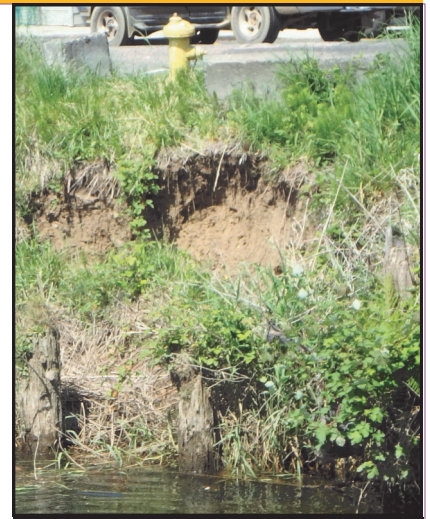
Clatskanie River extreme streambank erosion at 4th Street in Clatskanie.
