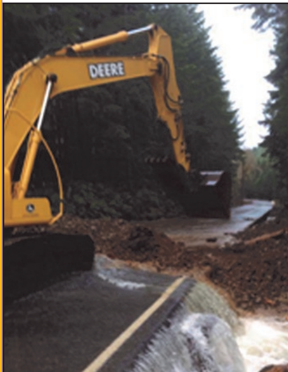
Archibald crossing on Apiary Road during flood event on December 11, 2015.
