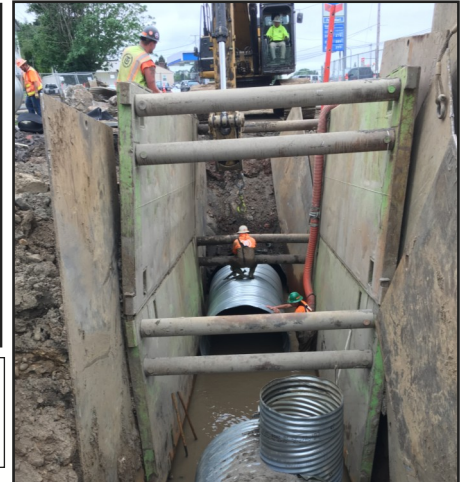
Right: Crews replacing sections of the pipe inside the enormous sinkhole stabilized by large shoring boxes.
