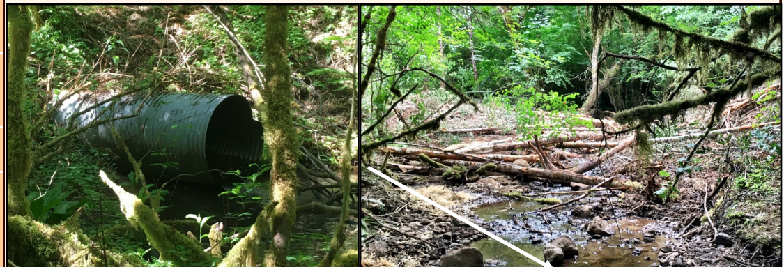
Before: A small, perched culvert conveyed Dribble Creek under the logging road creating a year round fish passage barrier.
